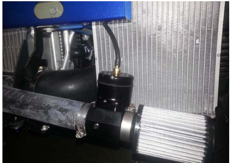
Vacuum Line Connected at Surge Valve
